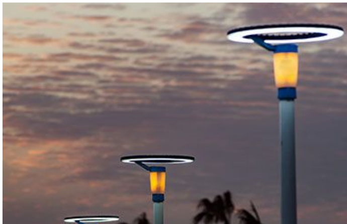
Solar powered street lighting
